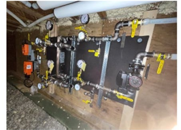
Figure 4 – Piping Manifold Installed
