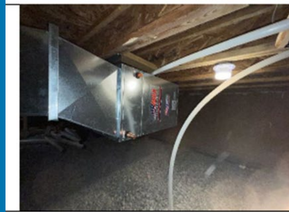
Figure 1 – Air Handling Units Installed
